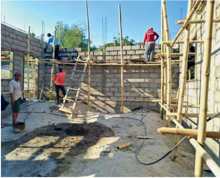
This building is going up with funds from NAC SEA Relief Fund (NAC South-East Asia)
